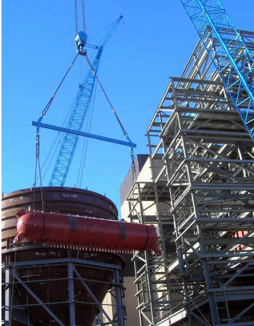
Workers at the Wygen III construction site at the Neil Simpson Complex raised the newly arrived steam drum into place on January 17, 2009.
